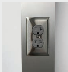
Electrical Outlets - pg. 26
